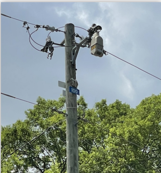
FIGURE 2. A TripSaver II recloser installed on Alabama Power’s lateral line.
