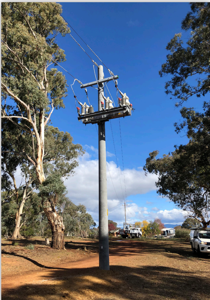
FIGURE 2. An IntelliRupter fault interrupter deployed on an Evoenergy feeder in a bushfire-prone area.
